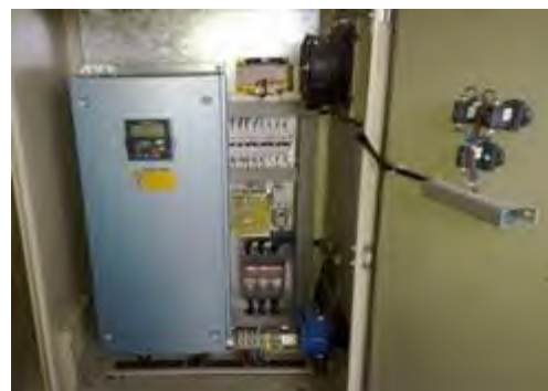
Figure 3. Frequency converter used in series connected pumps
