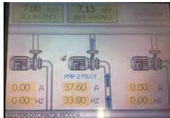
Figure 5. PLC used in an irrigation pumping plant
